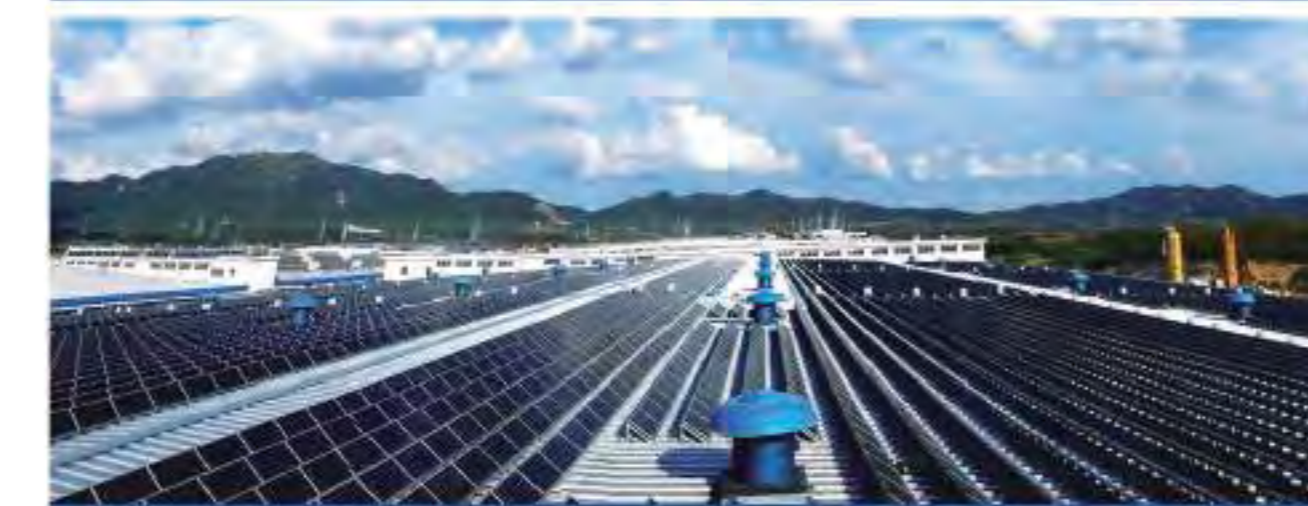
Solar panels arrays
